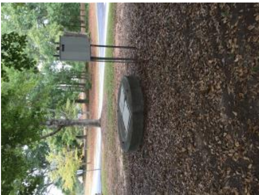
Sanitary lift station sump hatch is not secured. Sump is at least 20 feet deep.
