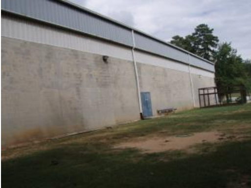
CMU Wall Requires Cleaning
