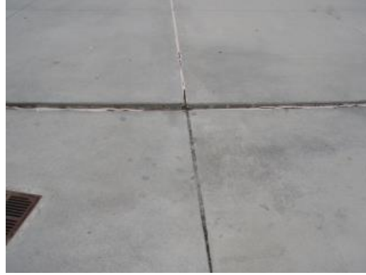
Uneven Surface Between Pools
